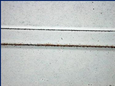
Figure 1. Red rust on tension bends of prepainted HDG.
