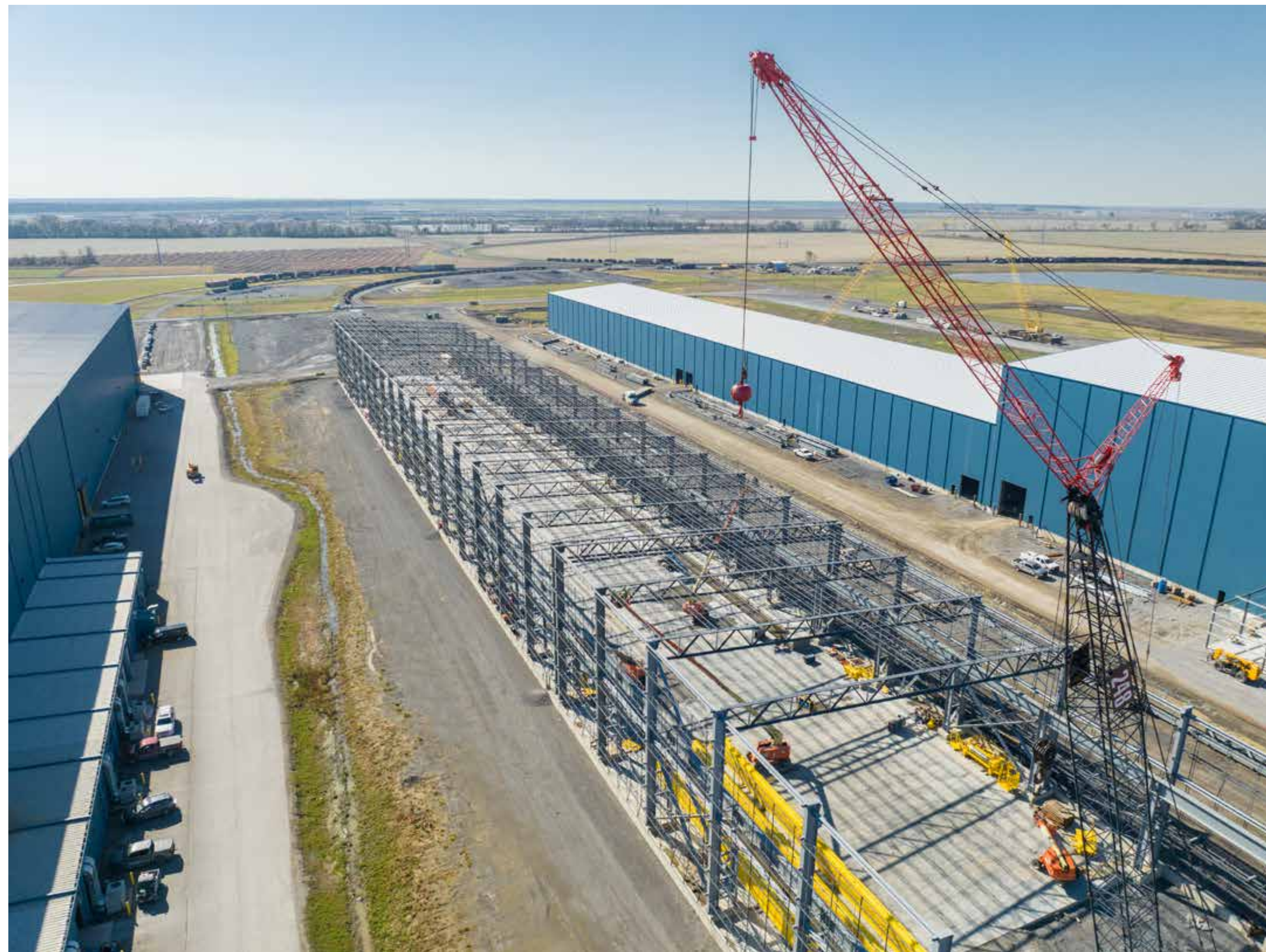
Construction of our new mini mill, Big River Steel 2, in Osceola, Arkansas.
