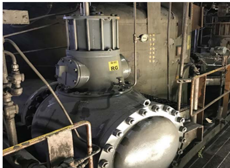
Figure 20. Clairton Switching Valve
