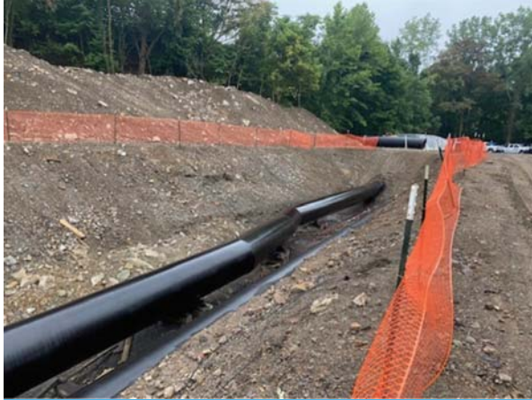
Figure 20. Coke Oven Gas Transport Lines
