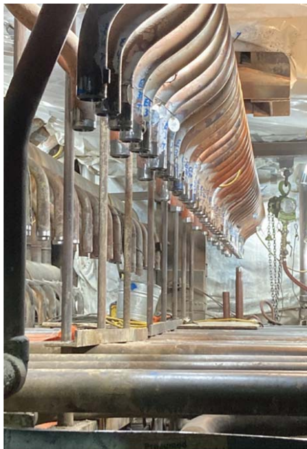
Figure XX. No. 2 Boiler Superheater Tubes
